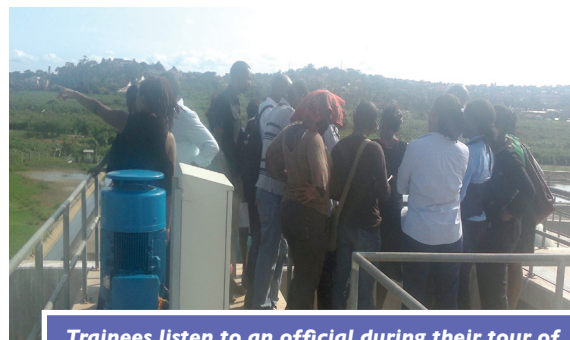
Trainees listen to an official during their tour of Bugolobi Sewerage Treatment Plant
